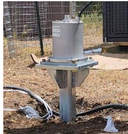
Coupled with Earth All vibrations pass through (Houston Test Site) 4,200lb version
